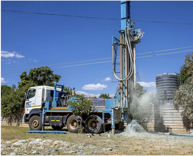
Groundwater Abstraction and related water reticulation Infrastructure
